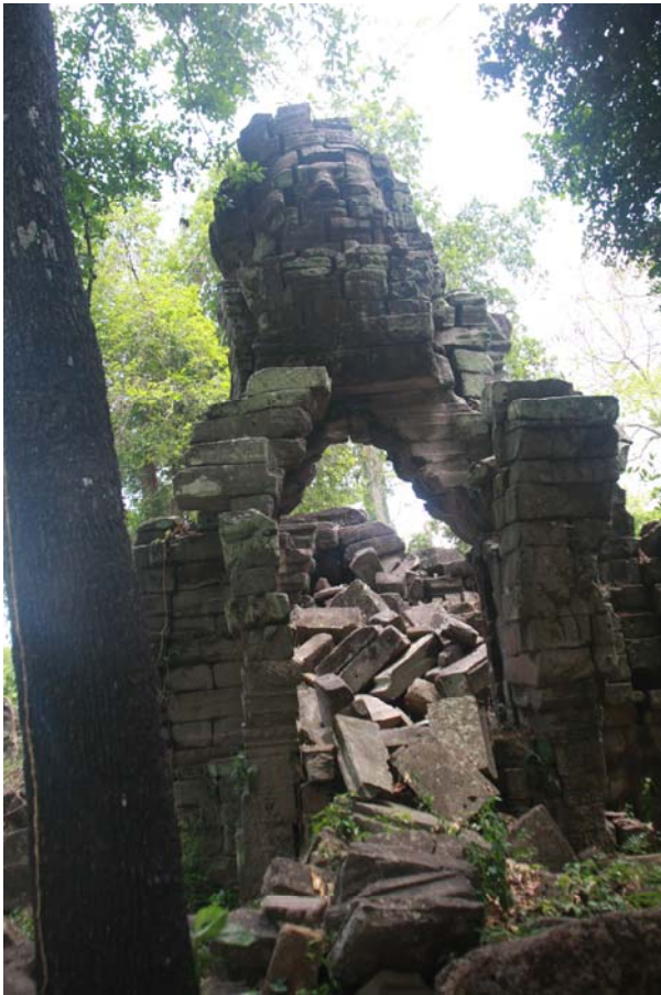
Most parts of Banteay Chhmar Temple collapsed or in the process of collapse (May 9, 2014)
