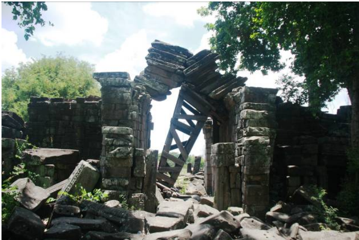
A collapsed part of Banteay Chhmar Temple is reinforced by wood structure (May 9, 2014)
