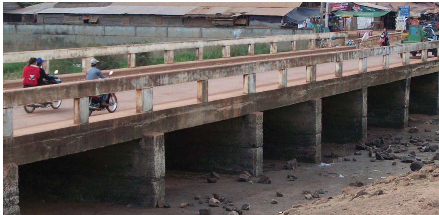
Built in 1995, Ta Mok ordered the construction of the bridge to facilitate transportation between Anlong Veng and Thailand. It is situated along the road from Anlong Veng to the Thai border checkpoint of Chaom Sra Ngam. To build this bridge, machinery was brought from Thailand. Source: Documentation Center of Cambodia Archives.
